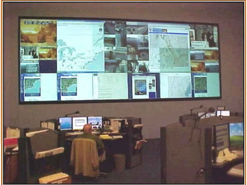
Traffic Management Center, Concord
